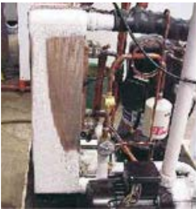
Figure 6.17a Thermo camera picture visualizing refrigerant mal distribution in a BPHE without distribution device. Photo of the same phenomena visualized by ice deposit on outside of the BPHE.
